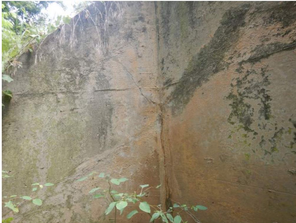
Photo No. 9 - Vertical crack in corner of northwest wingwall and headwall
