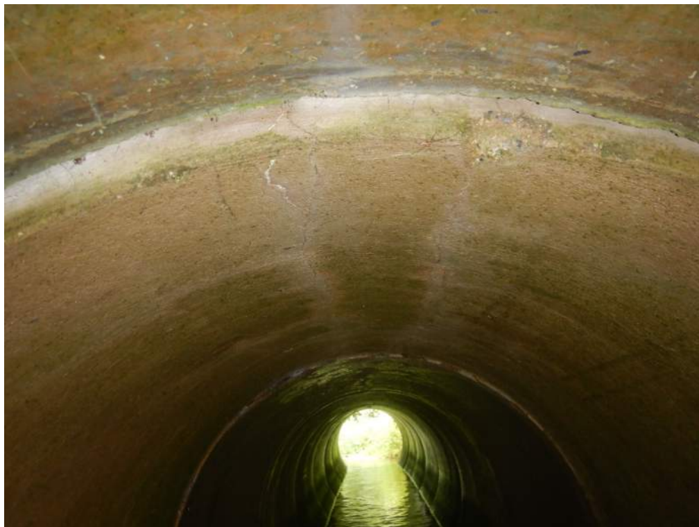
Photo No. 8 - Typical hairline crack
